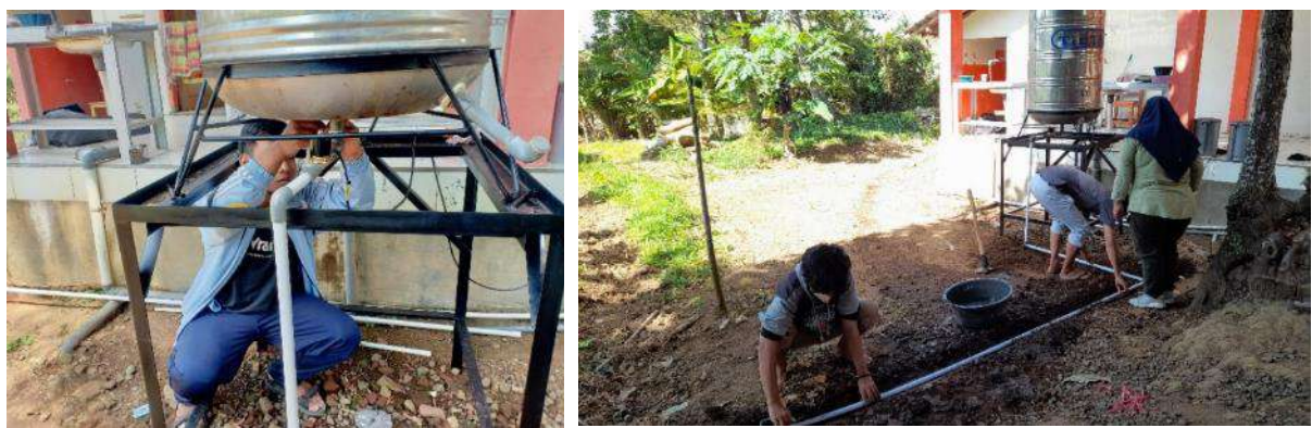
Figure 3. Drip irrigation system (a) automatic timer installation (b) soil excavation for irrigation pipelines
