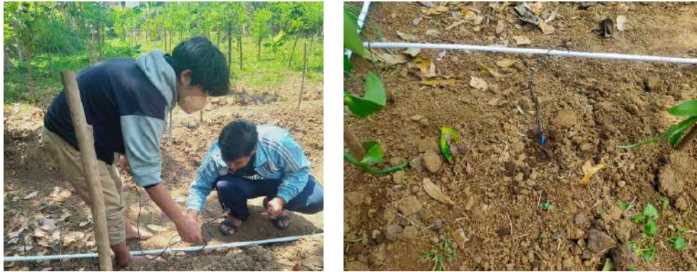
Figure 4. Drip irrigation assembly
