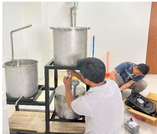
Fig. 5. Assembly of essential oil distillation equipment by the supplier
