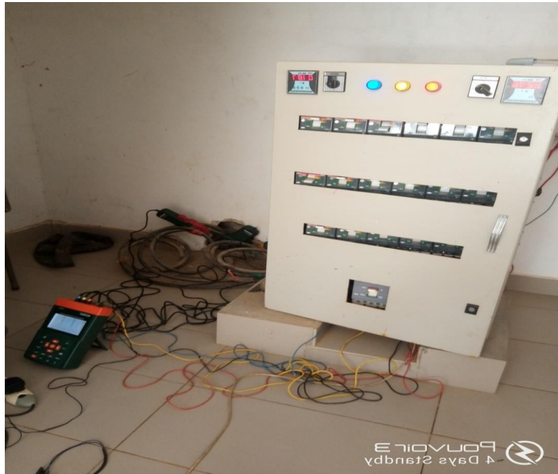
Figure 3. Power system analyzer connected with the distribution board
